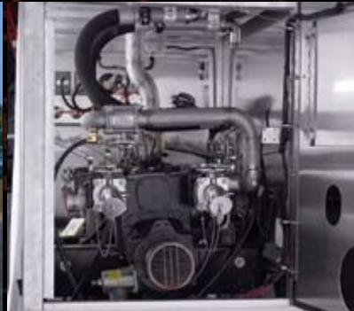
Full access to pump house
